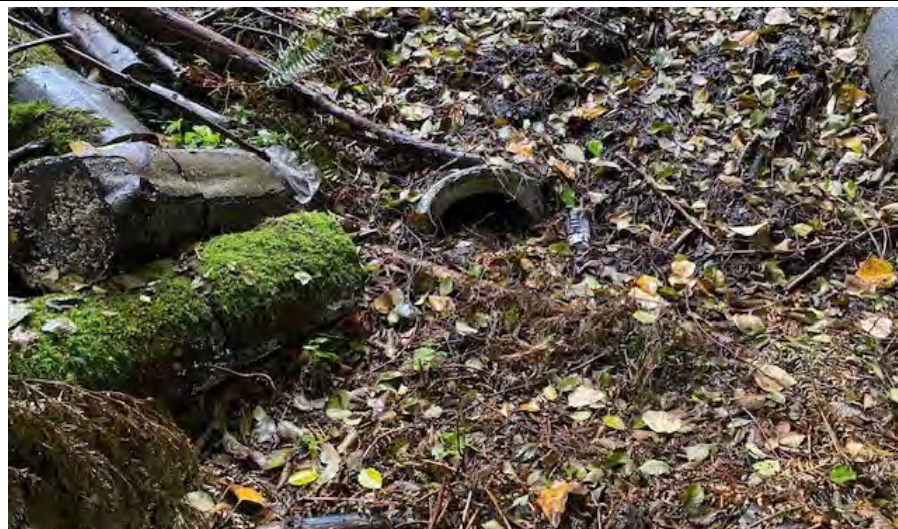
Photo 38 shows the culvert under Bond Road in the upland between Bond and Stottlemeyer Roads in the south segment.
