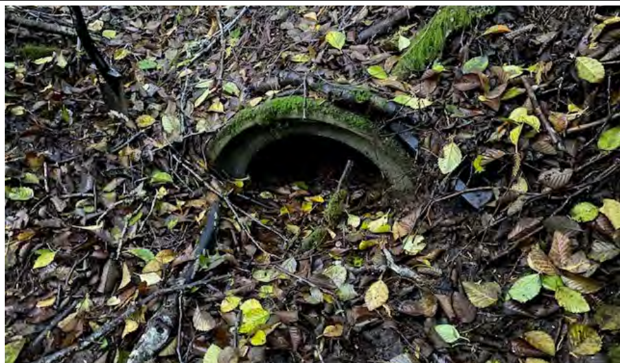
Photo 37 -Shows the inlet of the culvert under Stottlemeyer Road, which is at the end of the non mapped stream just west of the road.
