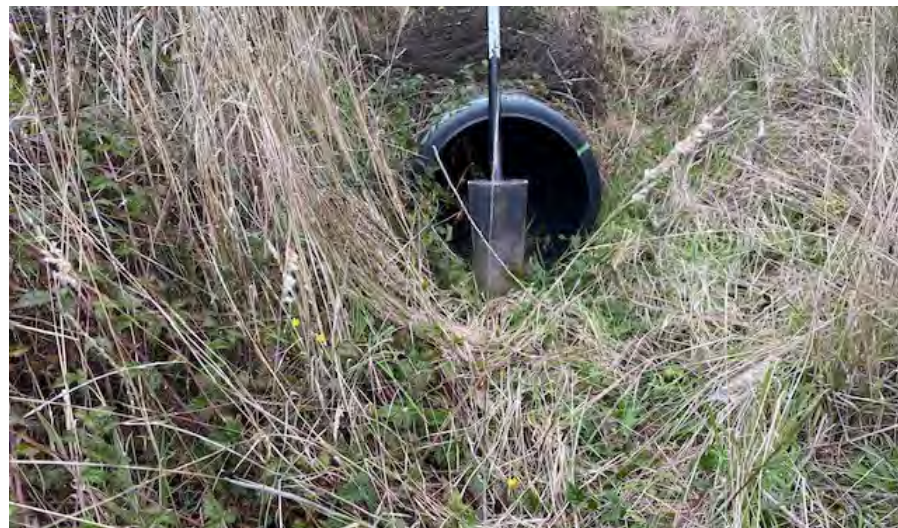
Photo 40 shows a culvert under one of the service road. It appears that the culvert was installed during construction of logging roads.
