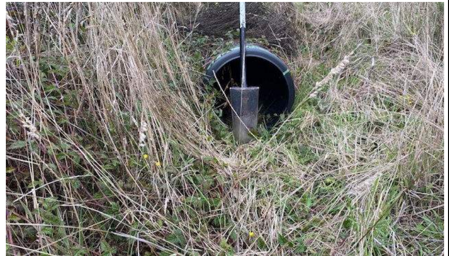
Photo 36 shows a culvert under one of the service road. It appears that the culvert was installed during construction of logging roads.
