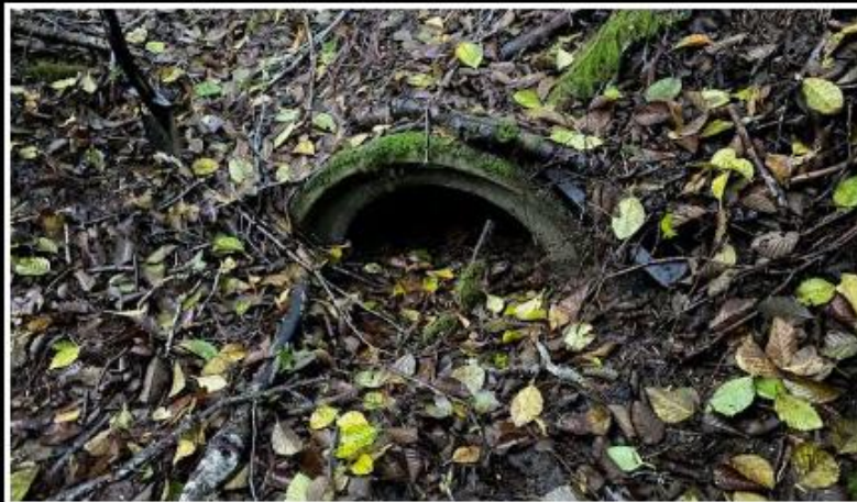
Photo 33 -Shows the inlet of the culvert under Stottlemeyer Road, which is at the end of the non mapped stream just west of the road.
